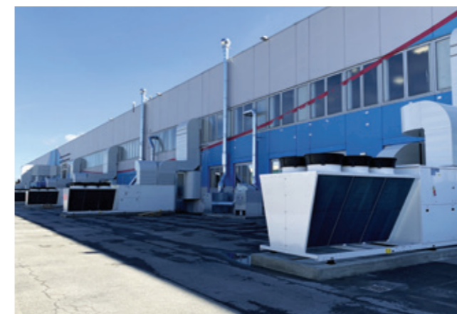
Figure 10: Example industrial production facility installation ©Clivet
